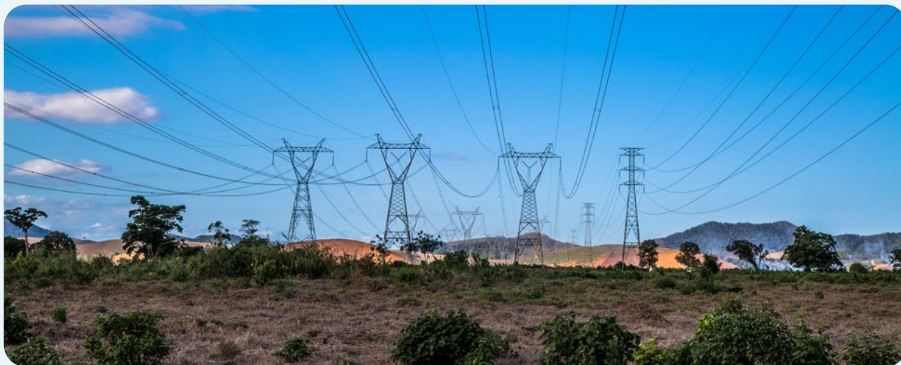
Macaé-Campos Transmission Lines I, II and III. Photo: Daniela Monteiro
