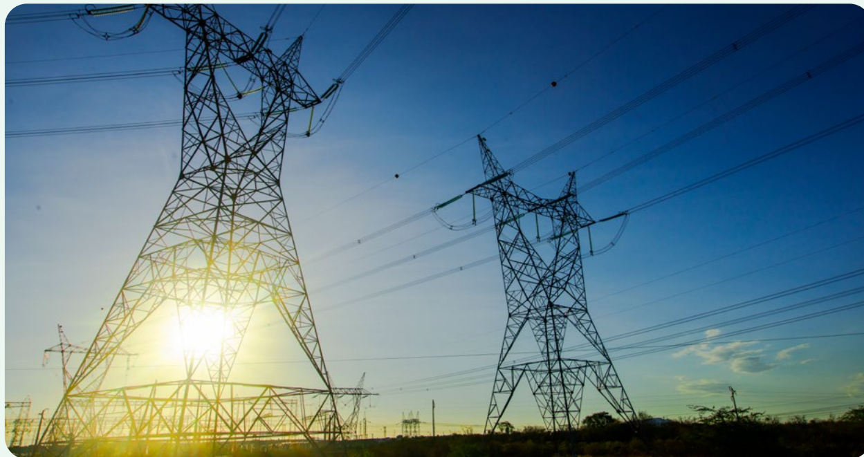
Eletrobras Chesf transmission lines. Photo: André Schuler
