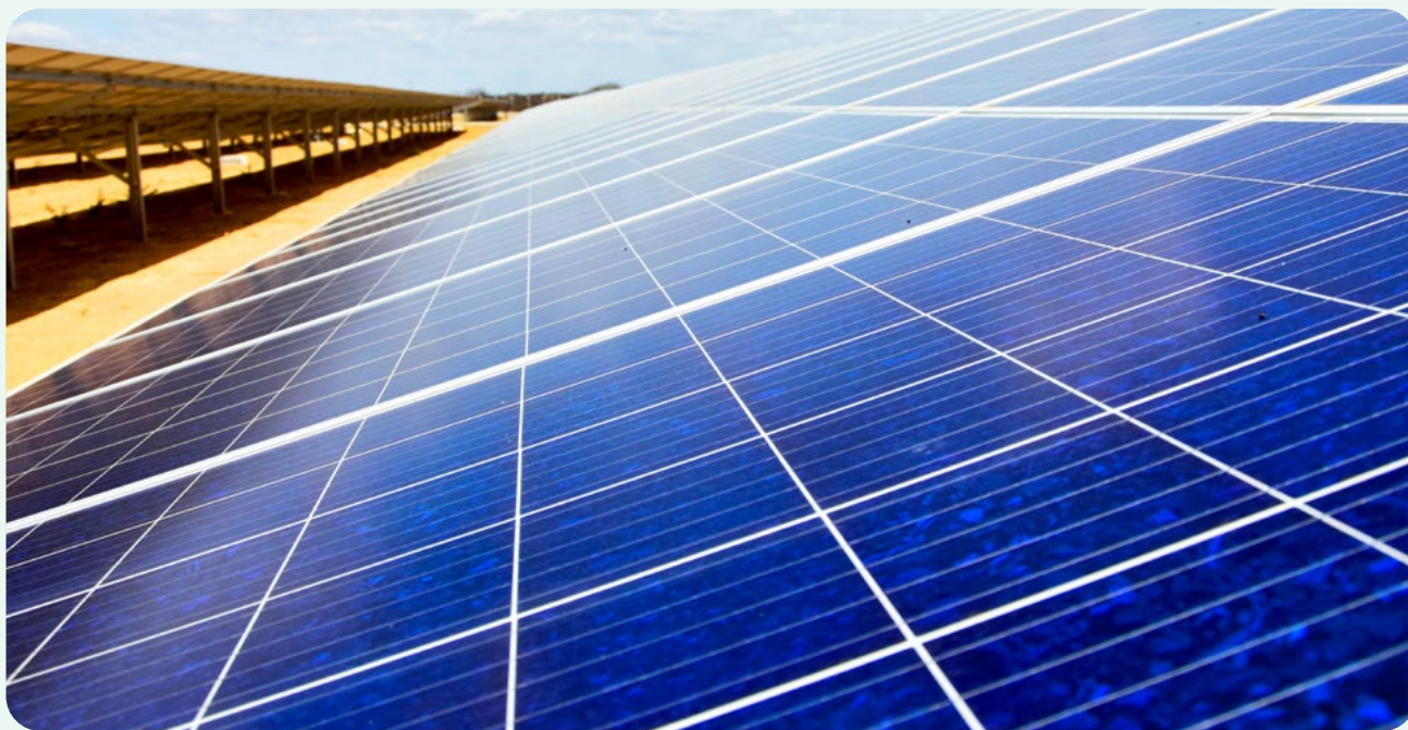
CRESP (Pernambuco Solar Power Center of Excellence). Chesf Archives
