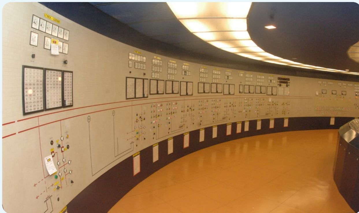
A control panel at Chesf. Photo: Chesf Archives
